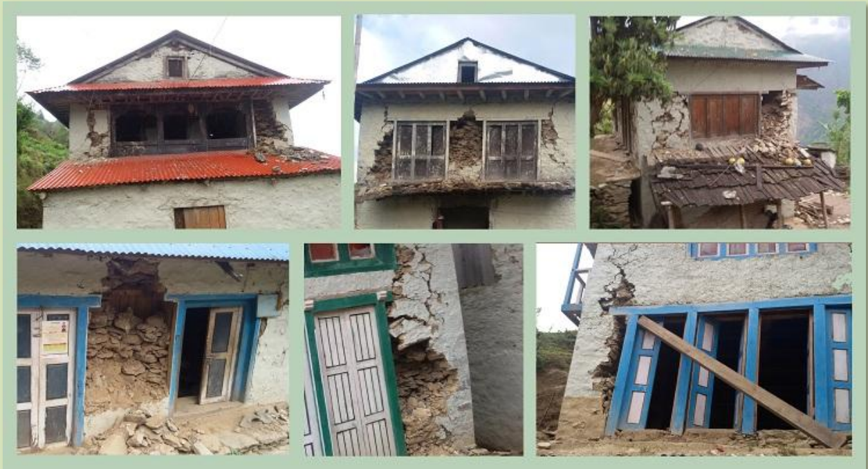
Pictures of some of the damaged houses throughout Rapchha
