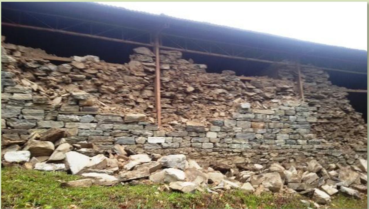
Damaged wall of the Secondary school
