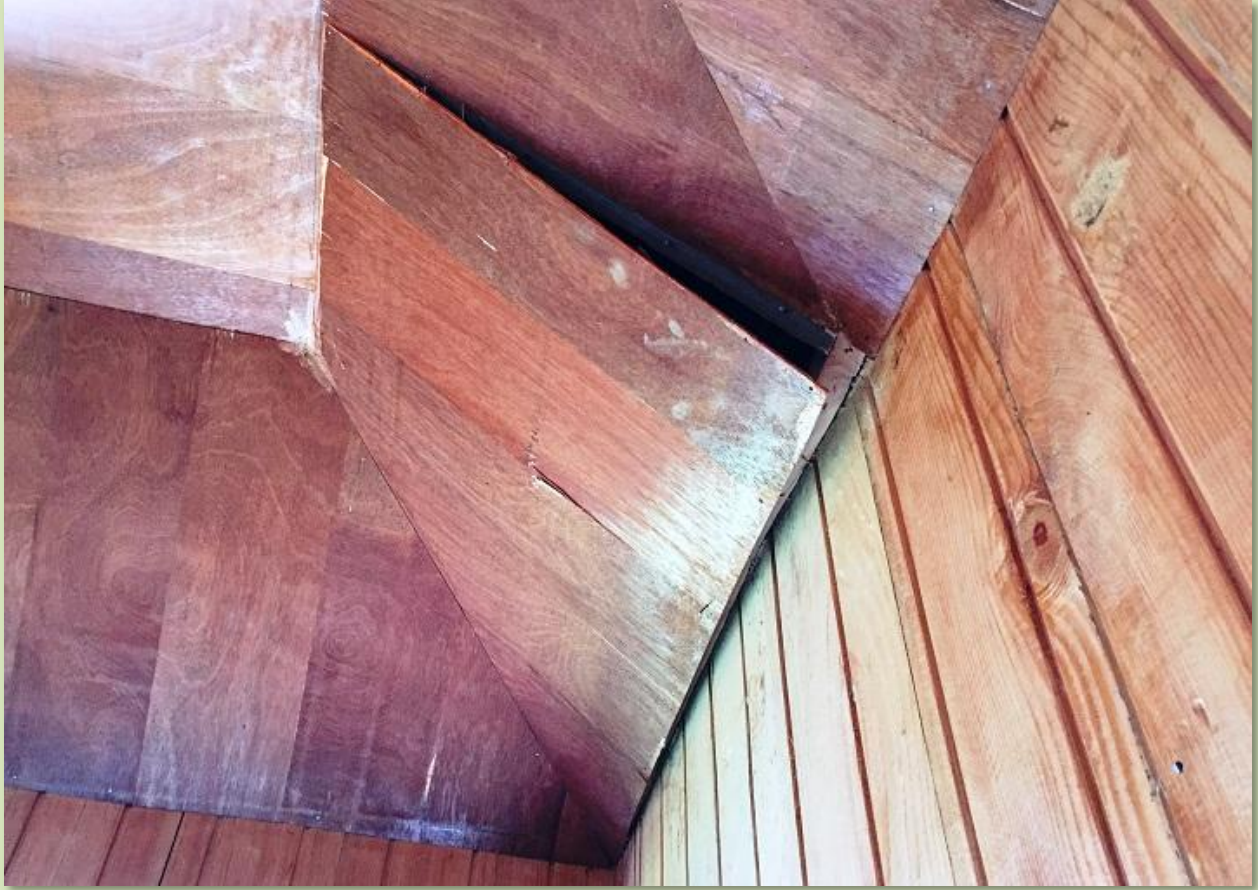
A broken ply on the ceiling of a healthpost room (hit by fallen stone from the wall above)
