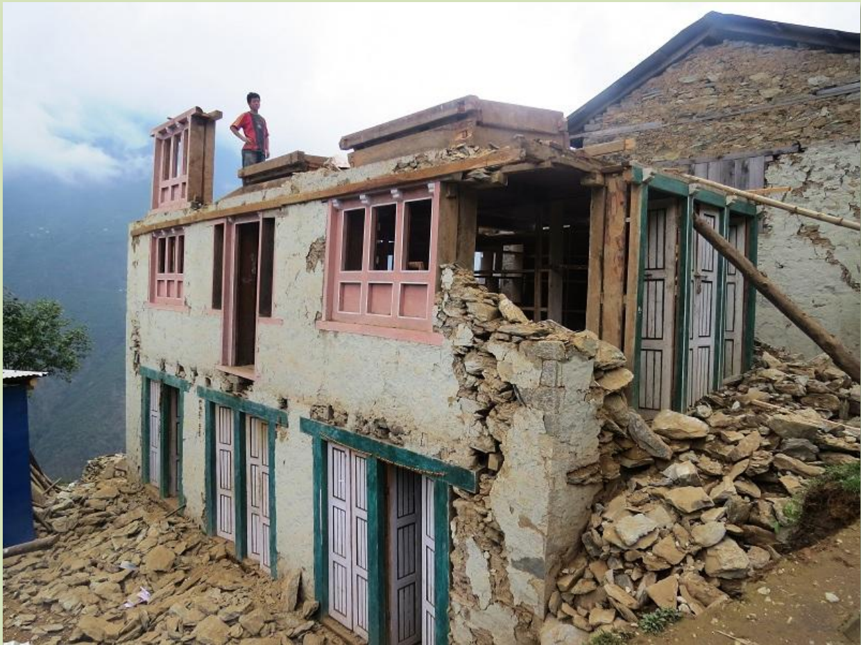
One of the damaged houses in Rapchha
